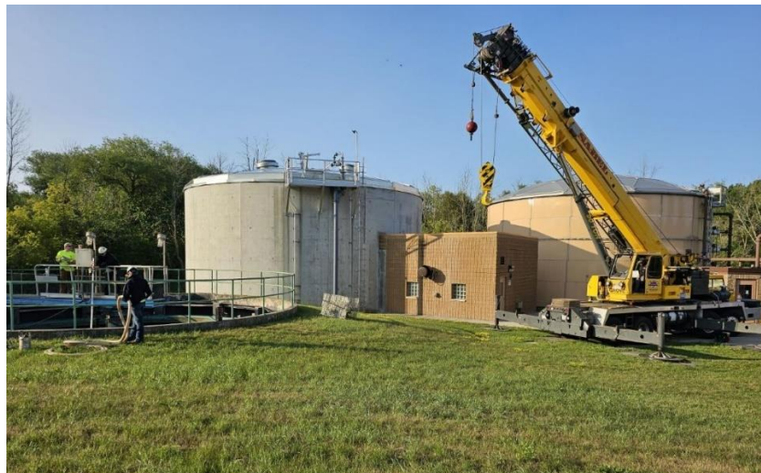
Village Wastewater Treatment Plant
